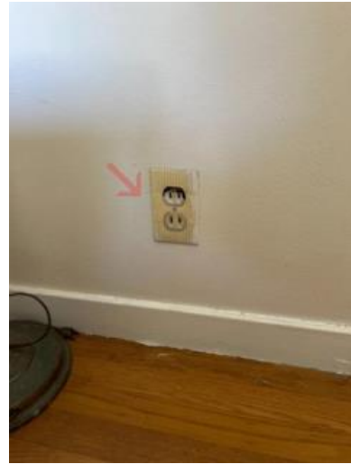
The accessible receptacles are functional and GFCI protected.
